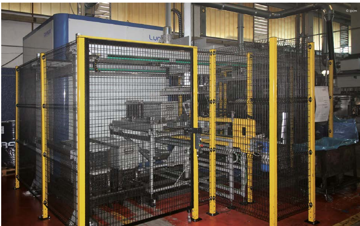
Cemastir's LUNA modified alcohol cleaning plant.
